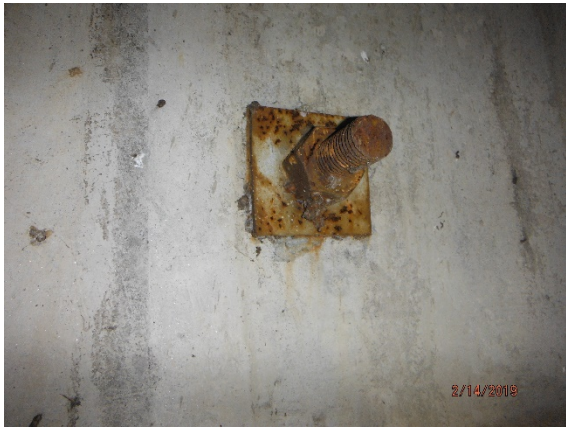
Photo 3. LBP Positive Tie Rod Plate
