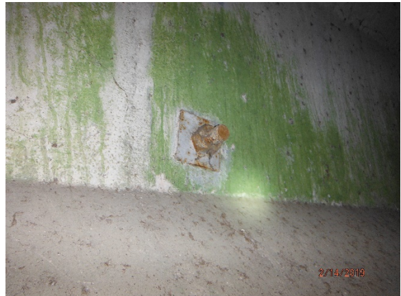
Photo 4. LBP Positive Tie Rod Plate
